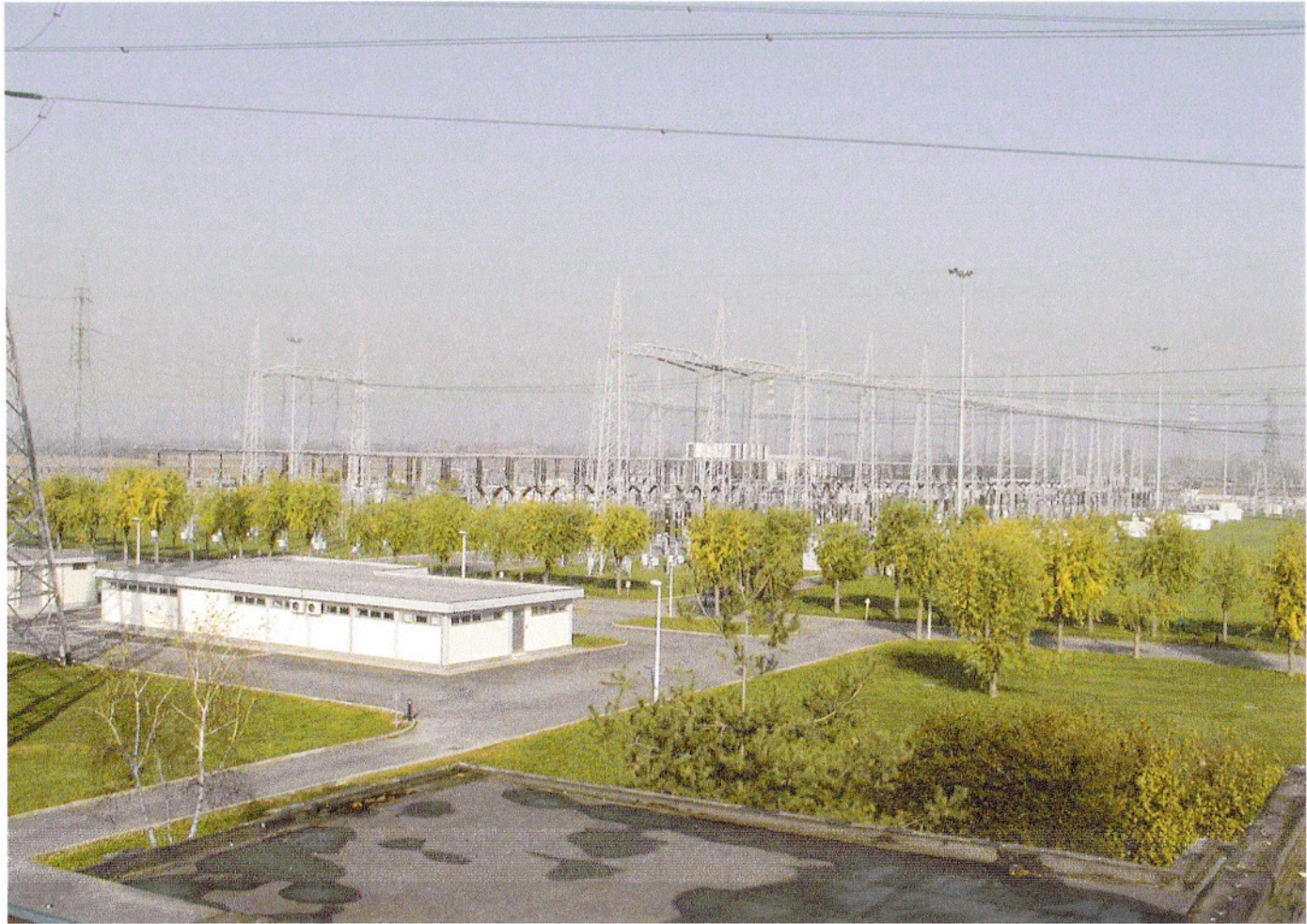
ENEL Center of Rondissone (courtesy of ENEL)
